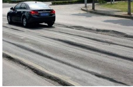
FIGURE 1: Rutting damage of pavement.
