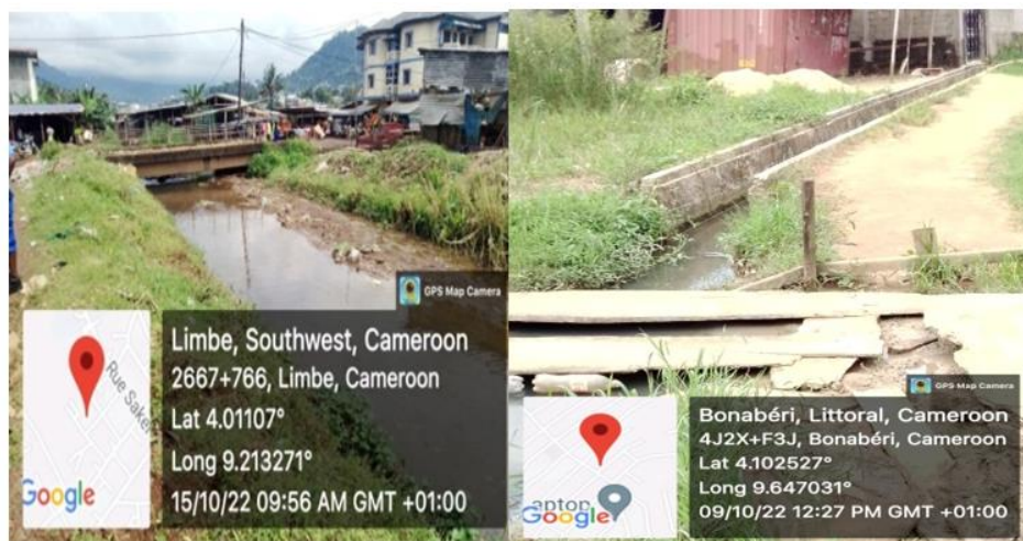
Plate 1. Engineering Drivers of Flooding in D4M and L1&3Ms
